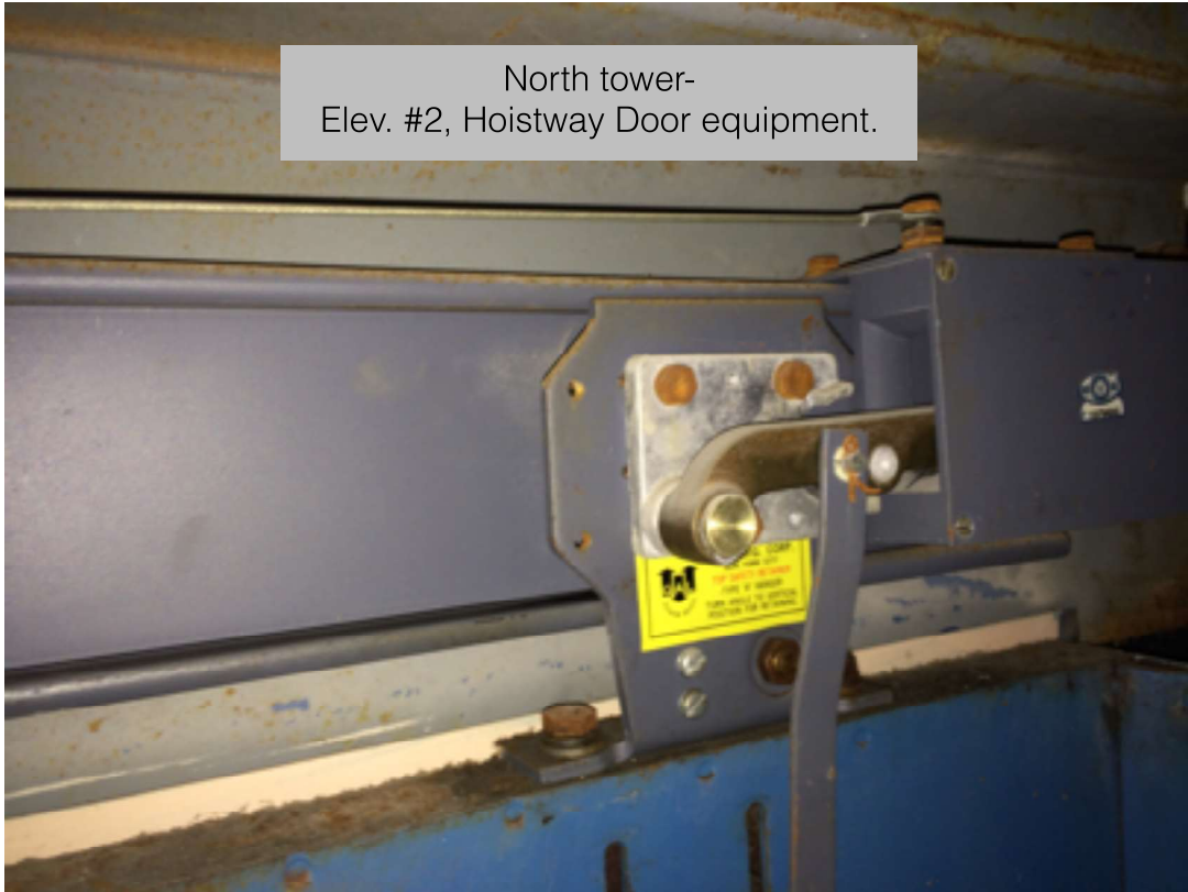
North Tower - Elev. #2, Hoistway Door equipment.
